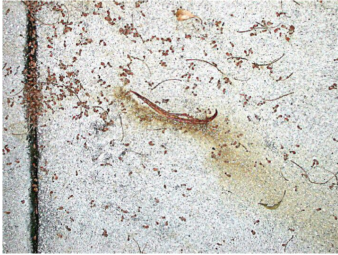
Fig. 2. The dark, rust stain on this sidewalk is associated with the string bean-like gall (center of picture) caused by eriophyid mites. Characoma nilotica larvae tunnel into the galls and their subsequent frass droppings cause the majority of the stain. Note there is no objectionable stain near the oxhorn bucida fruit (nutlets) in the crack of the sidewalk.
